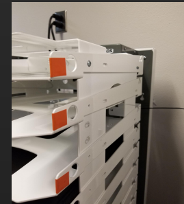
Figure 3) Colored stickers on each rack.
